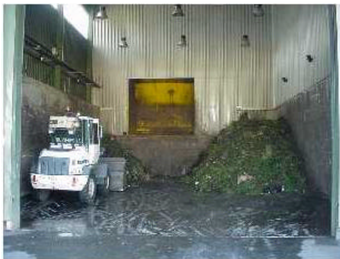
Figure 19: In vessel mixing and homogenisation facility for compost raw materials (separately collected biowaste) for Agricultural composting Plants
